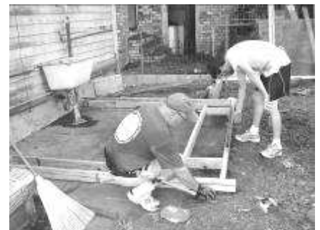
Ken and Jon working hard on the forms for the concrete footing.
