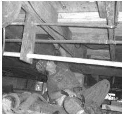
Alice, under the house, shoring up our shoring up efforts to shore the floor.
